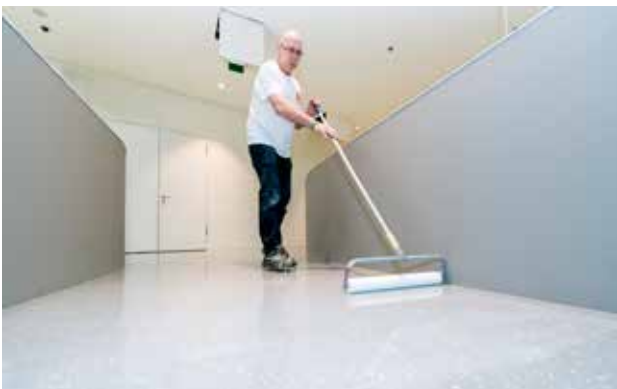
STEP 5. The finishing touch is the application of a transparent or pigmented topcoat. Typically this step involves a roller or spray application. The top coat secures the desired final design, and adds friction and wear resistance qualities to the buildup.
