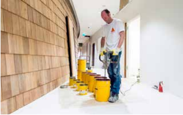
STEP 1. After inspection and preparation of the subfloor by cleaning (and if needed shotblasting, grinding, sanding and/or leveling), we will start mixing our liquid materials.
